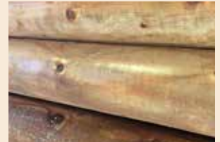
It has been difficult for brown colour to penetrate in packed posts.
